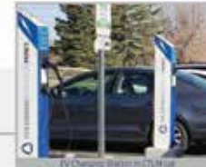
EV Charging Station in CTLM lot
